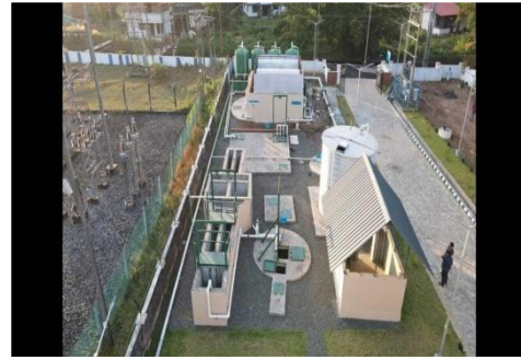
1 MLD CSTP at Padanappalam, Kannur
