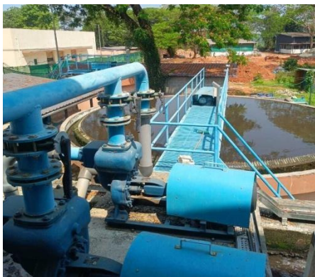
500 KLD STP at Kozhikode medical College
