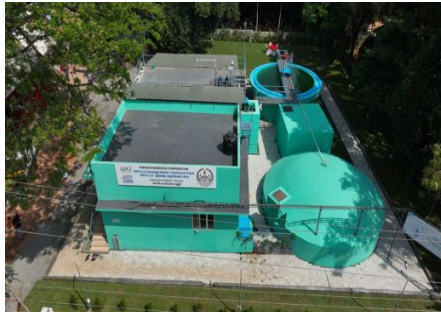
360 KLD STP at General Hospital, Thrissur
